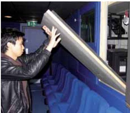
The projectors are mounted vertically in narrow compartments at the rear of the auditoria, with the beam angled through a 45 degree optical quality mirror. Access to the projectors for service purposes is gained via an easily opened hatch (above)
